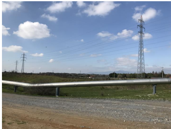
Photo 3-1. View of the Pipelines
